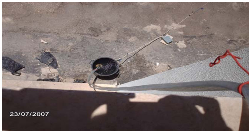
Figure (B.2) Submersible Pump inside the lower tank.
