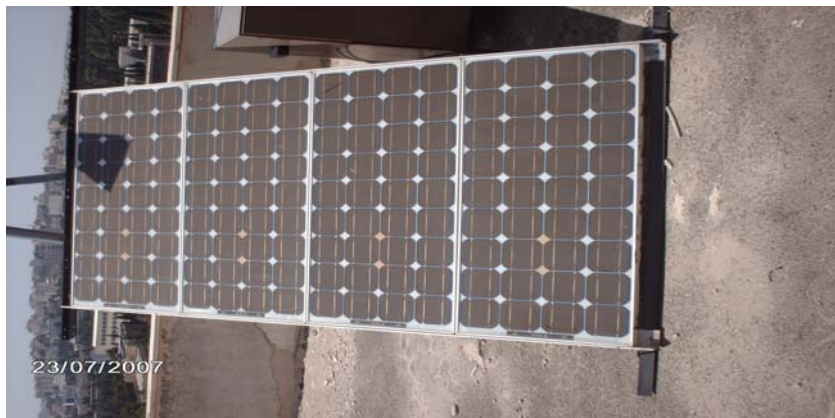
Figure (B.3) Photovoltaic panel of monocrystalline (four modules).
